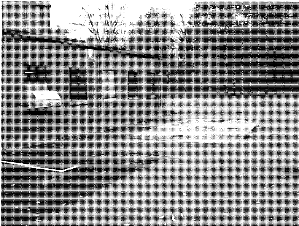
Foreground – Existing 5,000-Gallon Fuel Oil Underground Storage Tank Fills
