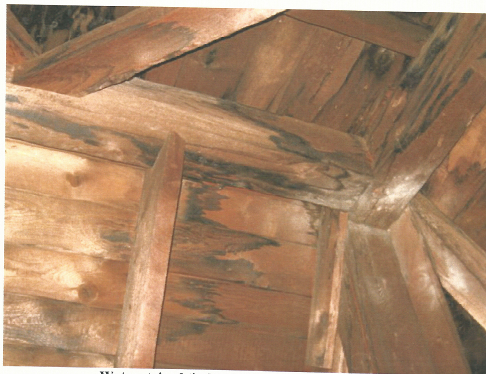
Water stained timber beams, roof joists and deck
