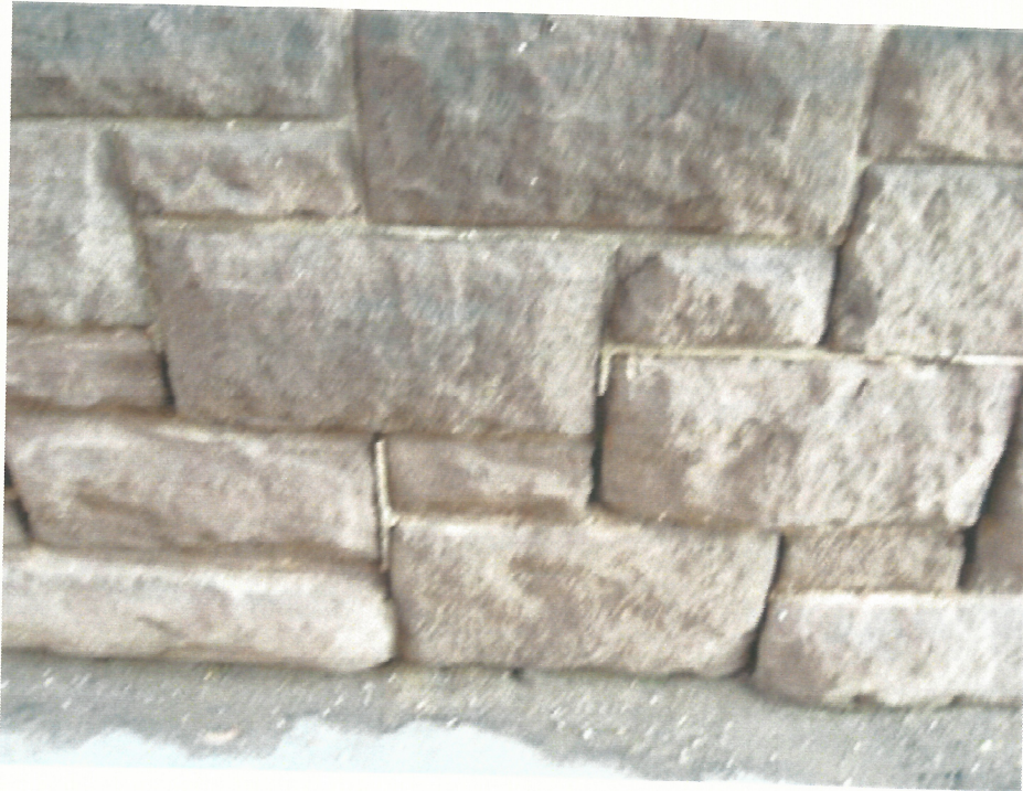
Spalling mortar in stone foundation wall mortar joints
