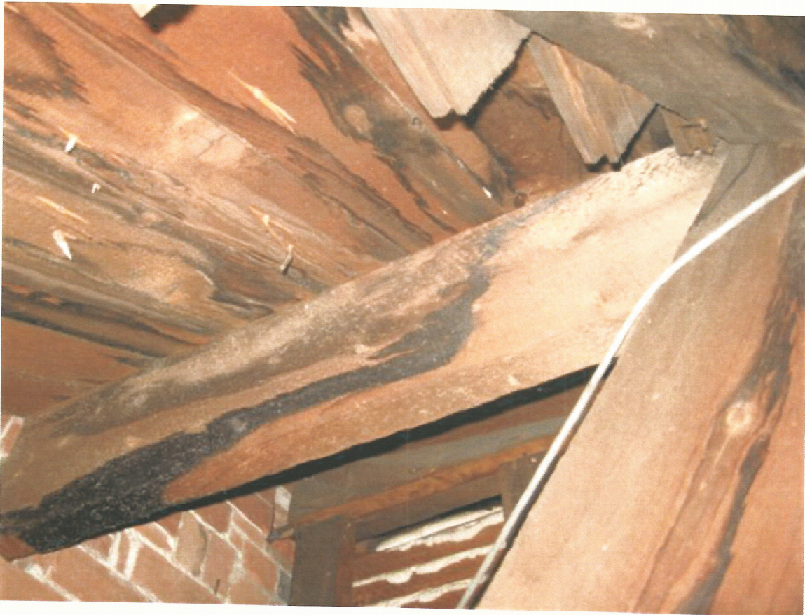
Water stained timber beams viewed from the Attic
