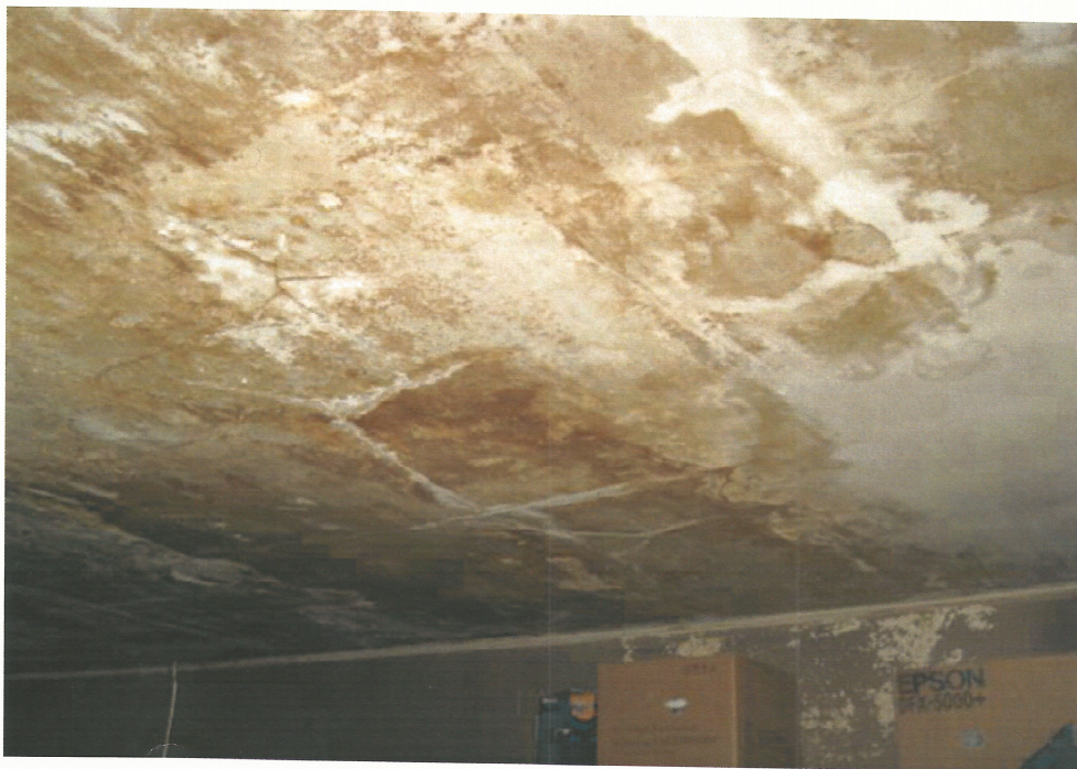
Water stained and sagging plaster ceiling viewed from the Third Floor
