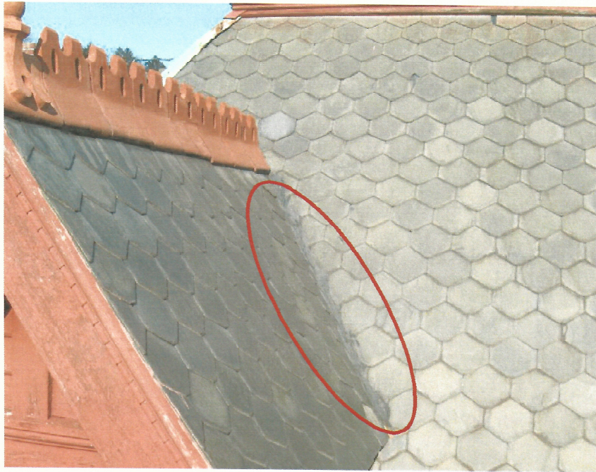
Copper Valley Flashing Covered with Roofing Cement
