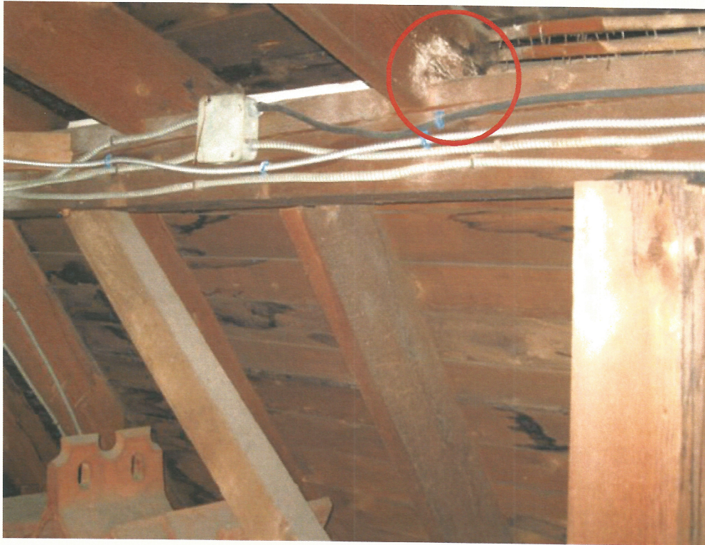
Water stained roof joist at bearing end
