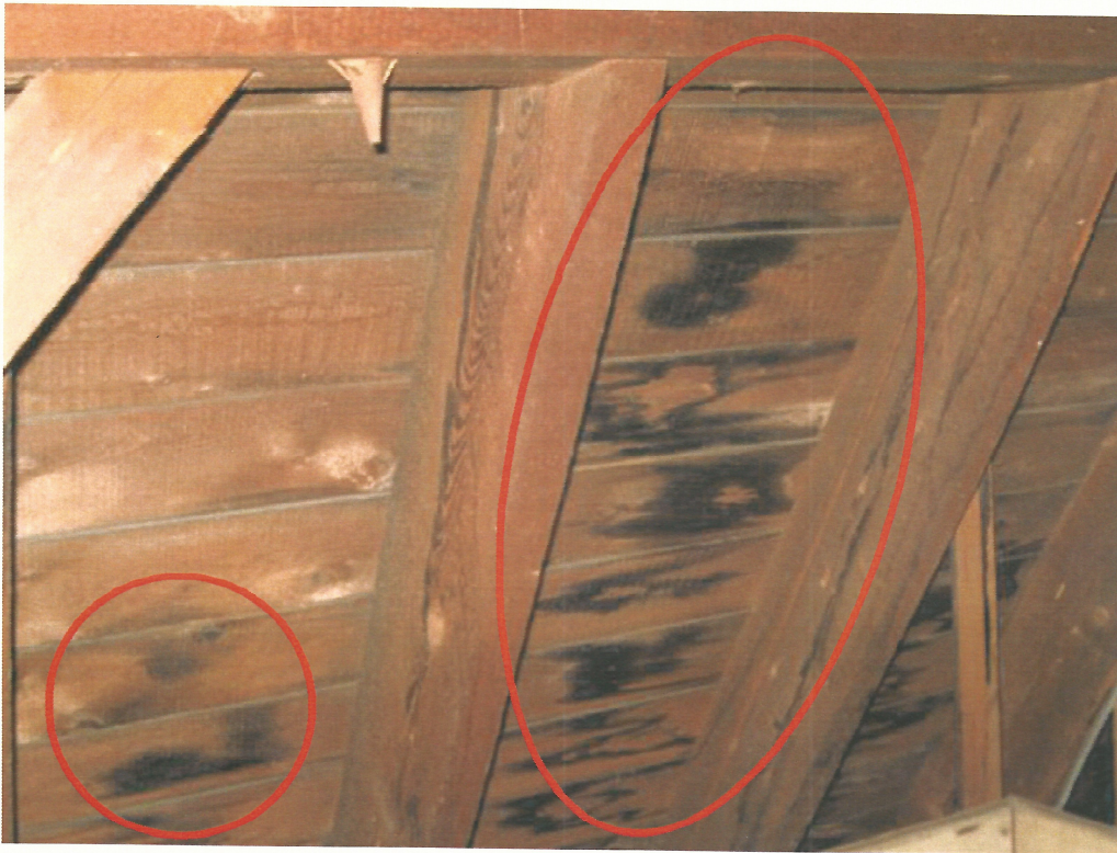
Water stained wood roof decking
