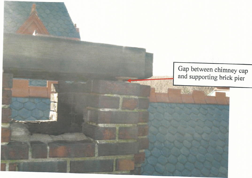
Close up of damage to the north chimney viewed looking south
