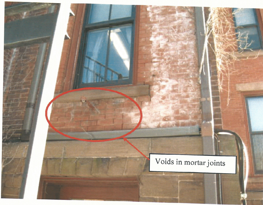
Close up of the efflorescence in the brick alongside the downspout
