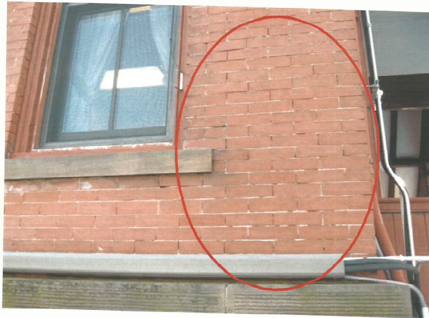
Voids in mortar joints
