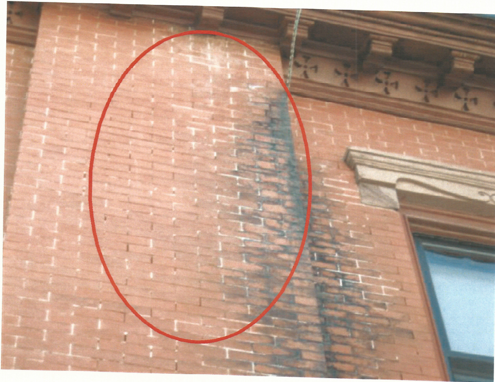
Voids in mortar joints and spalling mortar
