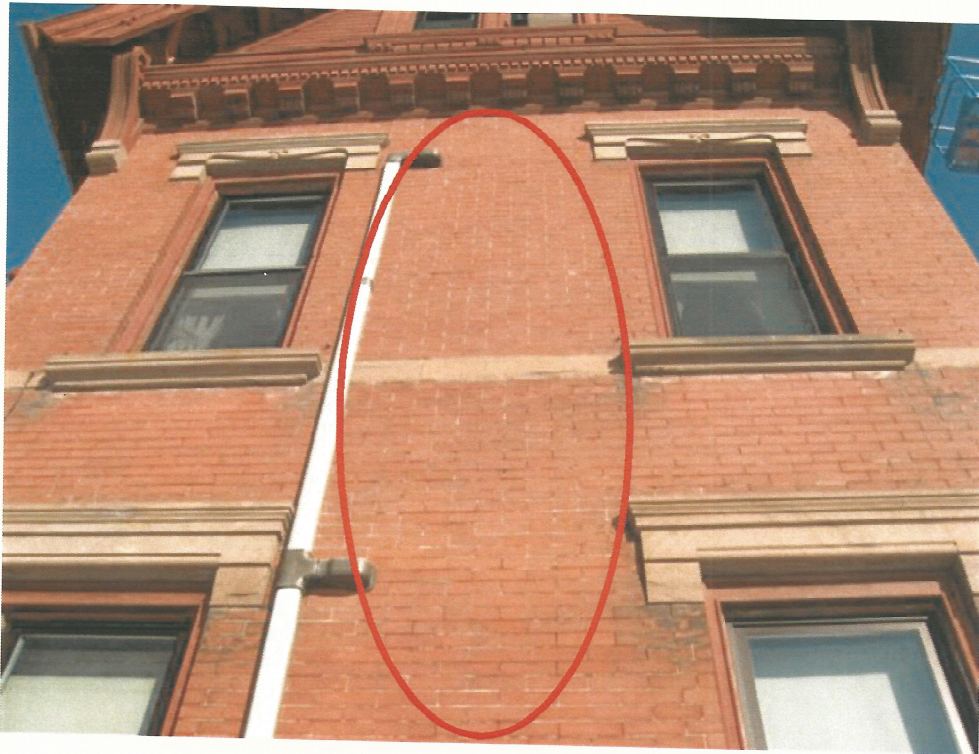
Voids and spalling in brick mortar joints
