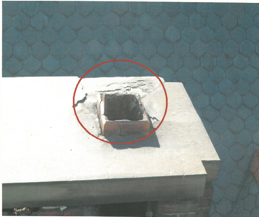
Damaged Chimney Cap
