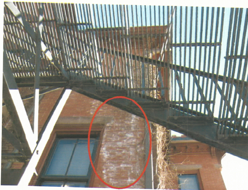
Efflorescence in brick at southwest corner
