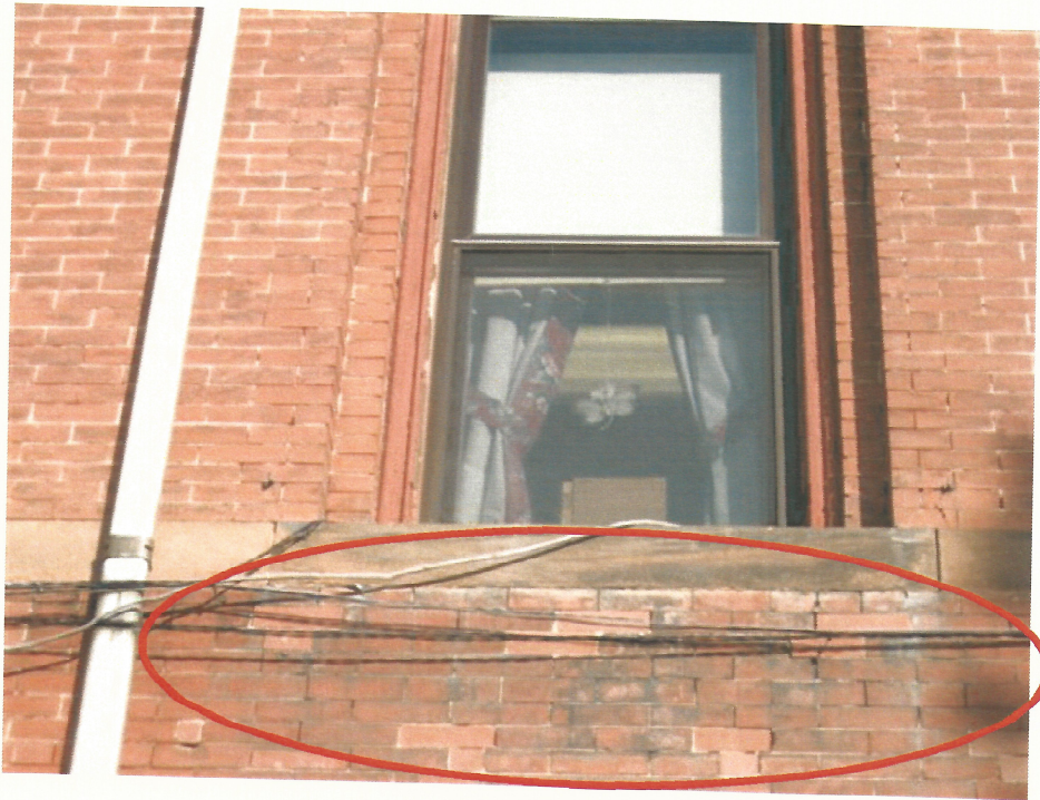
Failing masonry below window
