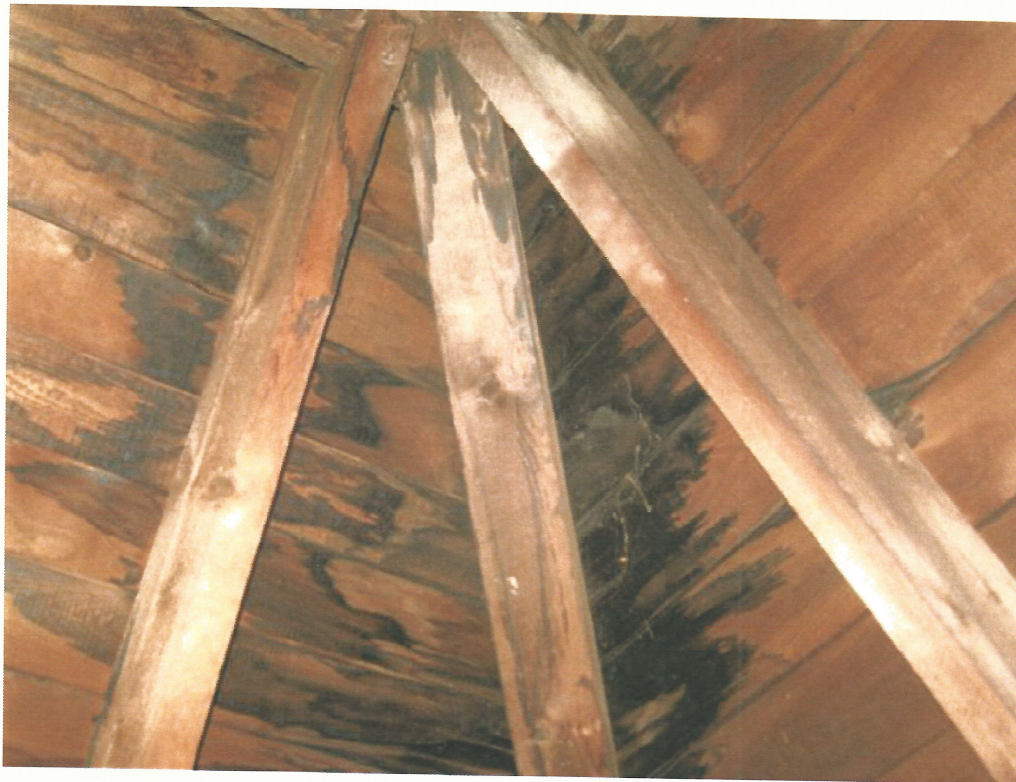
Water stained roof deck and timber beams at hip roof
