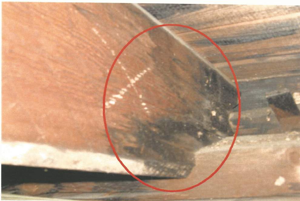
Water stained roof joist at bearing end
