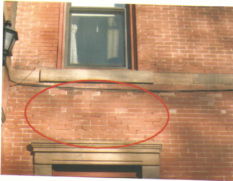
Movement above door opening with diagonal cracking
