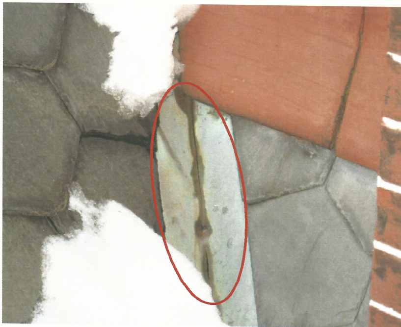
Copper Valley Flashing Spilt Open
