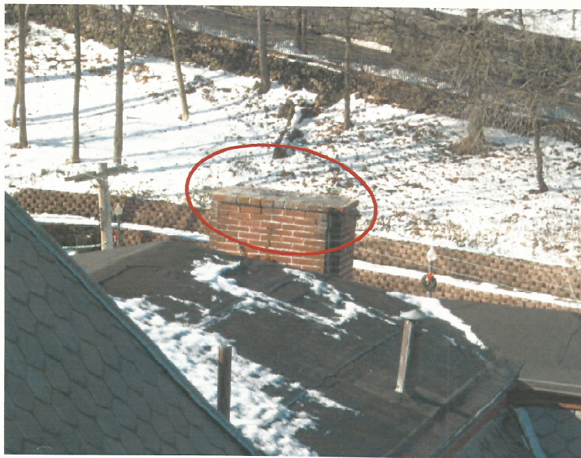
Missing Chimney Cap
