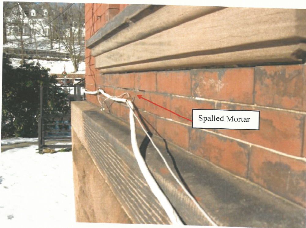
Spalling mortar joints in brick wall
