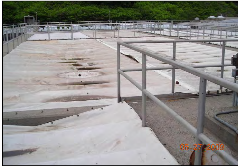
FIGURE 2-9 VIEW OF PRIMARY CLARIFIER COVERS FROM INLET END
