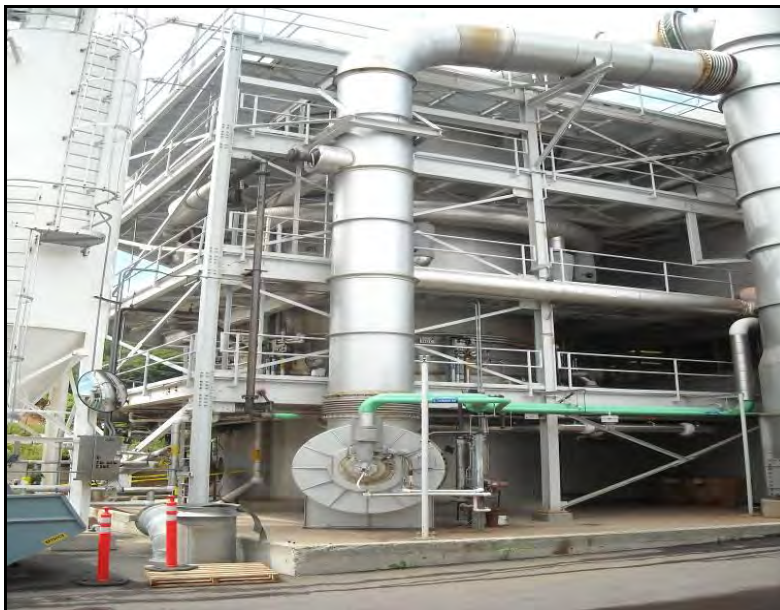
FIGURE 2-21 FLUIDIZED BED INCINERATOR
