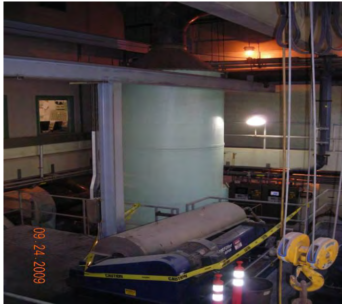
FIGURE 2-23 DEWATERING AREA SCRUBBER
