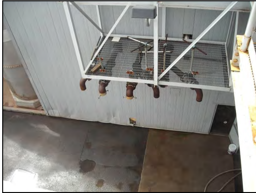
FIGURE 2-24 DEWATERED SLUDGE BYPASS PUMPING DISCHARGE STATION
