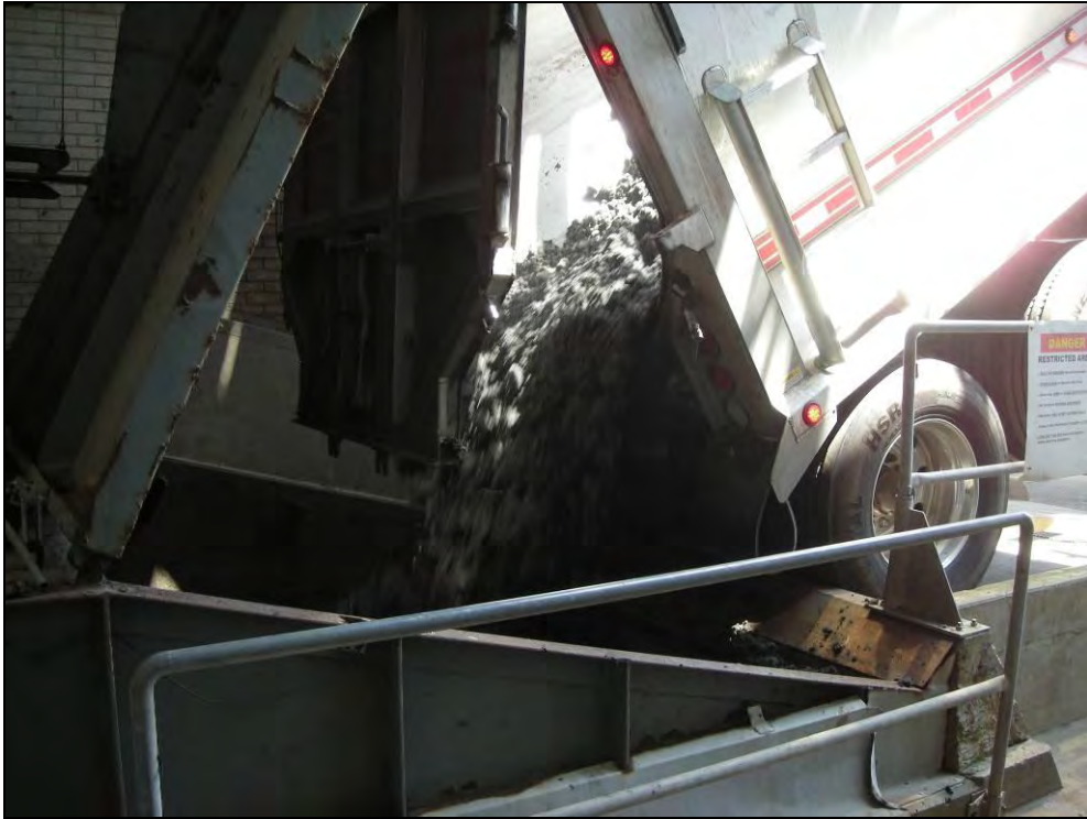
FIGURE 3-6 SLUDGE CAKE RECEIVING BIN
