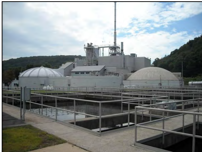
FIGURE 2-12 SECONDARY SETTLING TANKS WITH FILTER BUILDING IN THE BACKGROUND
