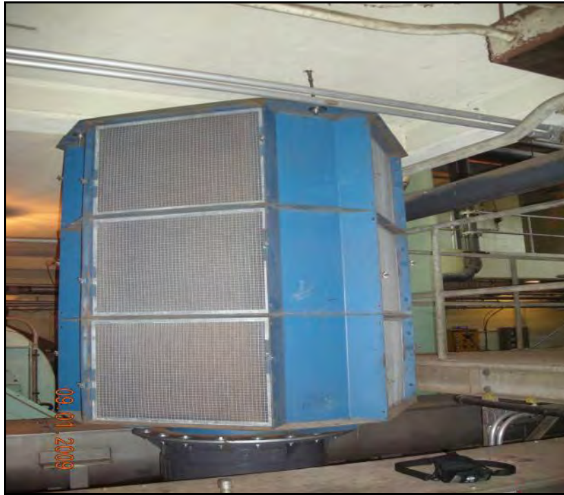
FIGURE 2-18 FLUIDIZED AIR BLOWER FAN EXHAUSTS FOUL AIR FROM DEWATERING ROOM TO FLUIDIZED BED INCINERATOR
