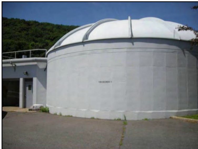
FIGURE 2-13 CIRCULAR THICKENER TANK WITH DOME COVER
