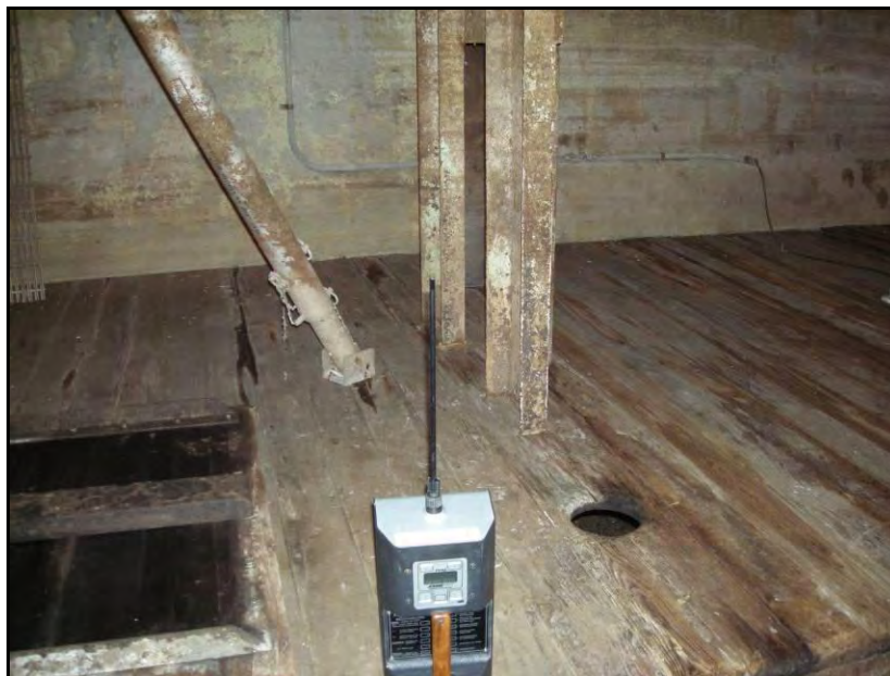
FIGURE 2-8 H2S MEASUREMENT IN THE WET WELL AREA
