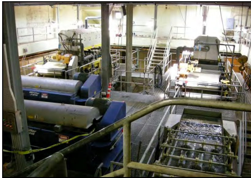
FIGURE 2-16 TWO BELT FILTER & CENTRIFUGE PASSES WITH A GRAVITY BELT THICKENER LOCATED IN THE FILTER BUILDING
