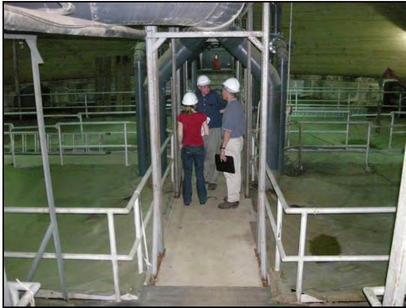
FIGURE 2-15 EXHAUST AIR EXHAUSTED FROM BELOW CLOTH COVER OF RECTANGULAR SLUDGE STORAGE TANKS
