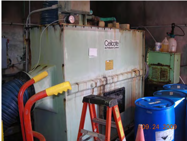
FIGURE 2-2 PRIMARY SETTLING TANK PACKED BED SCRUBBER
