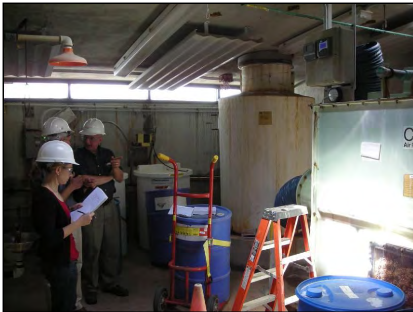
FIGURE 2-10 PRIMARY SETTLING TANK PACKED BED SCRUBBER
