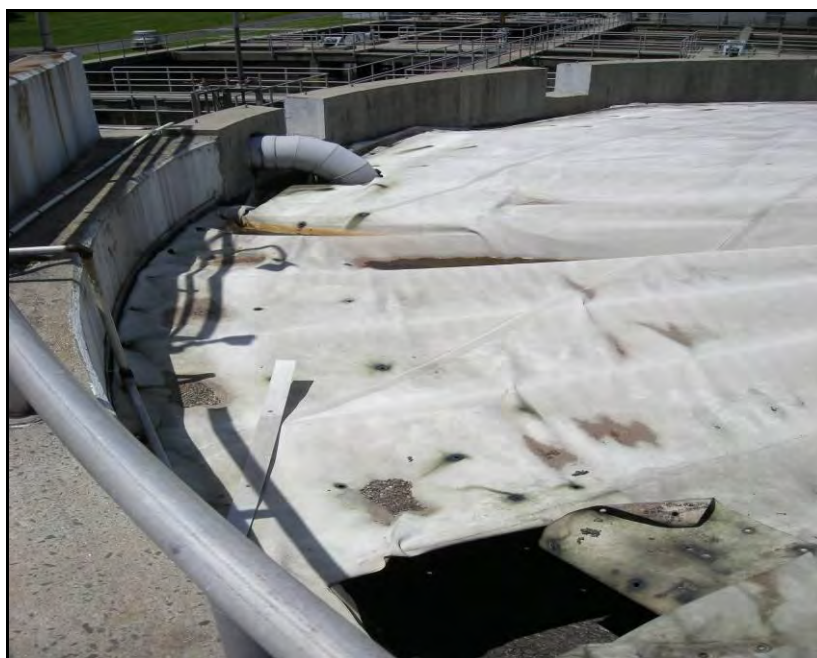
FIGURE 2-14 CIRCULAR SLUDGE STORAGE TANK WITH CLOTH COVER
